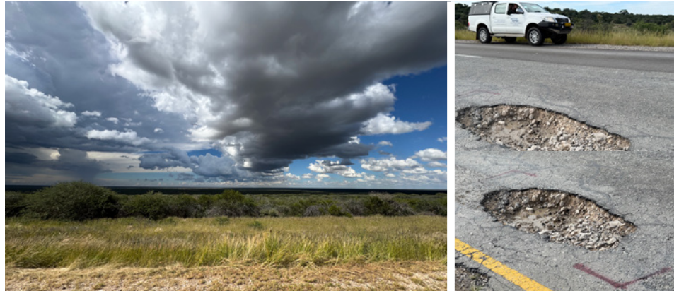
Fig. 25. Rainy season in Namibia: large and impressively deep potholes made driving tricky
