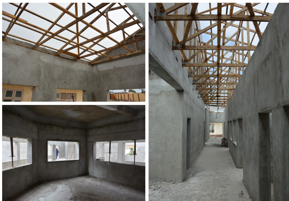
Fig. 4. The new neonatal unit in Swakopmund: the building is still in its shell, and it appears doubtful that it will be completed by the end of May 2023.
